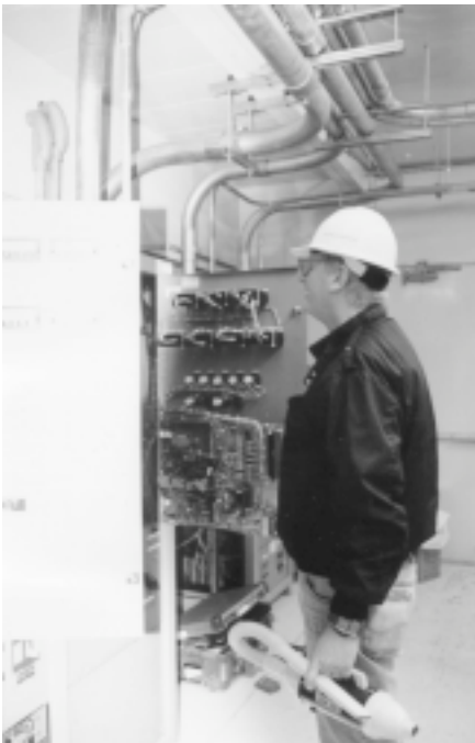
Solidstate Controls' start-up and commissioning service will assure a successful installation of your new power system. For more on this service, see "Money Saving Operating Tips" on the back cover.
